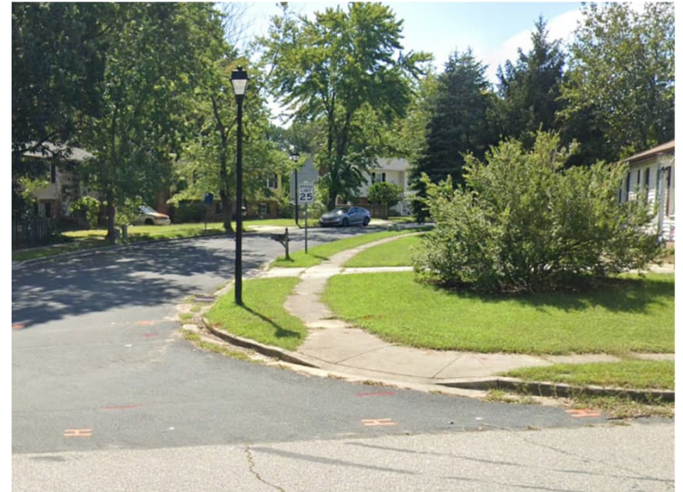
Sidewalk ramp ("ADA Ramp") does not meet standards
