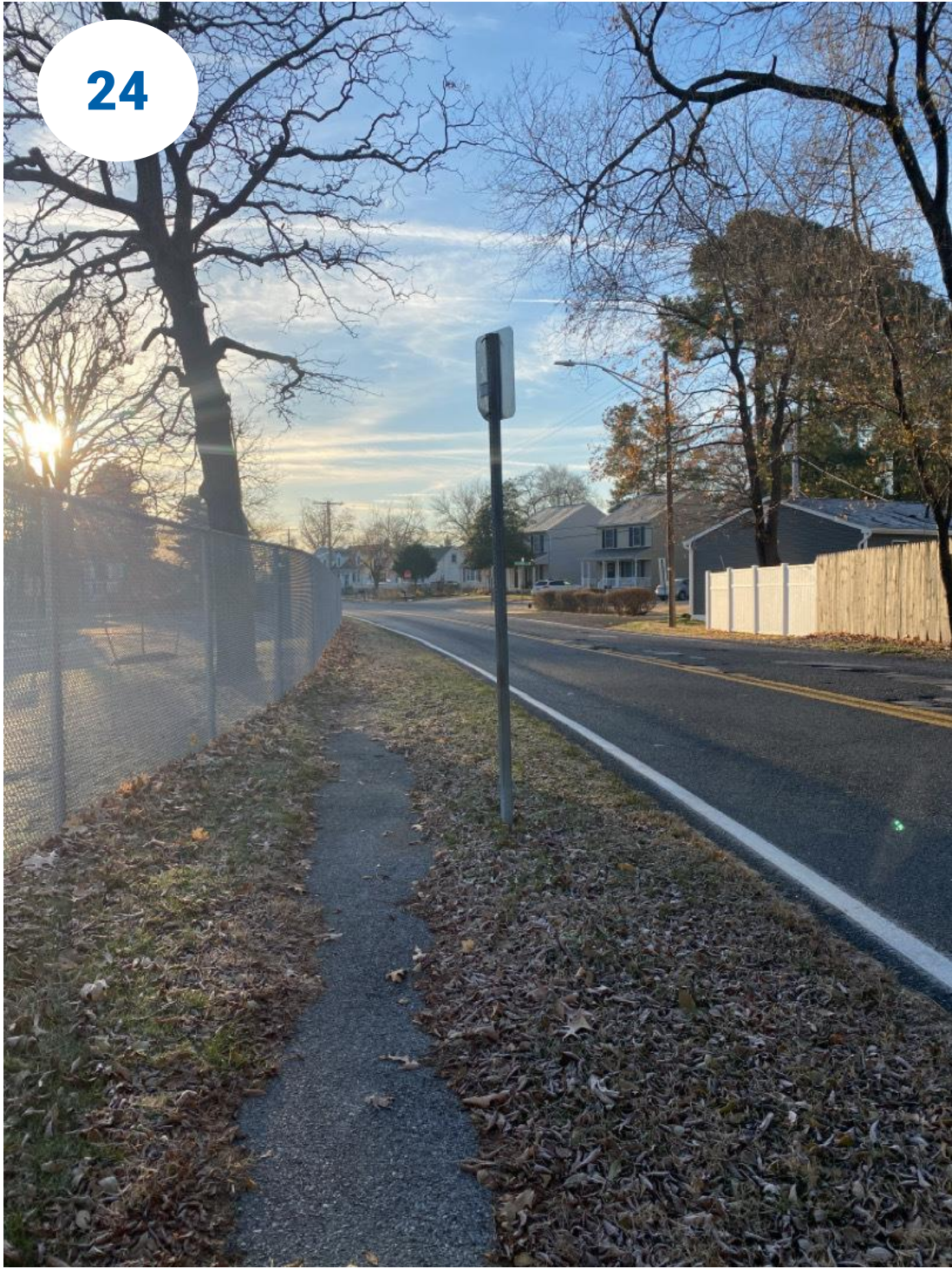
Condition of existing sidewalk on south side of 5 th Ave SW
