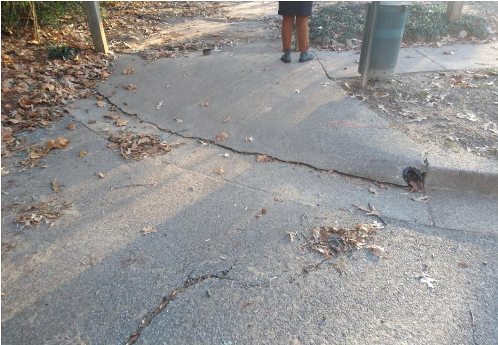
Greenhill Road at end of west sidewalk (top); Ramp to east sidewalk and trail toward Forked Creek Road (bottom)
